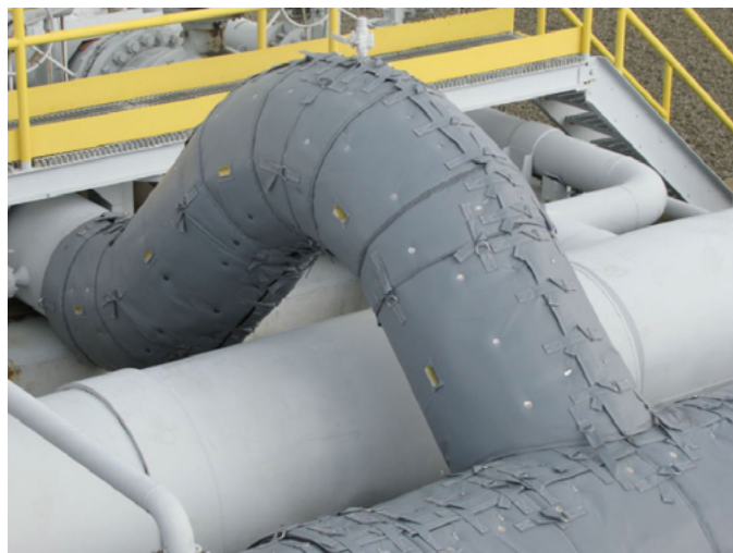
24" IPS Outdoor Service Piping – 12 dBA Reduction
