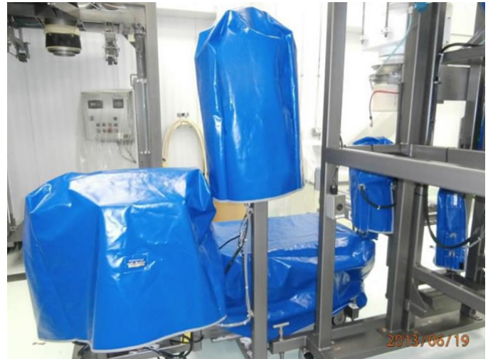
Production Wash Down Components (Motors, Terminal Boxes, Electronic Scale)
