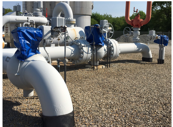
Gas Transmission Station Outdoor Valve Actuators
