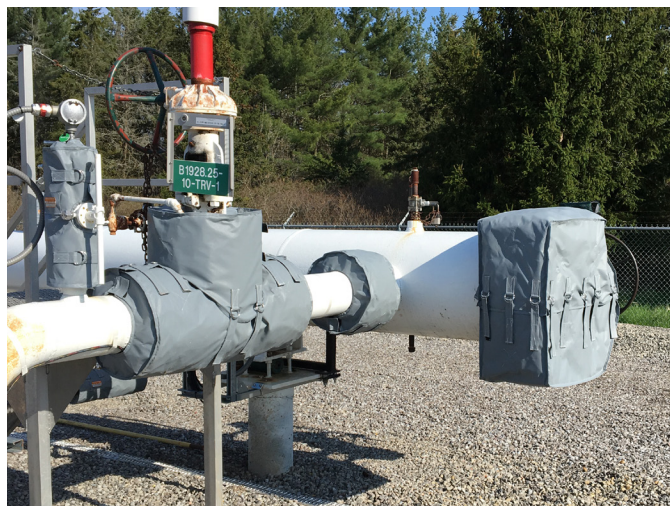
Pig Launcher / Process Valves / Flanges
