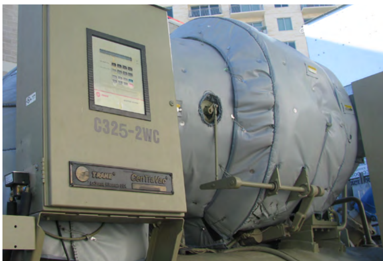
HVAC LIQUID CHILLER COMPRESSOR, COMPRESSOR INLET, MOTOR HOUSING
