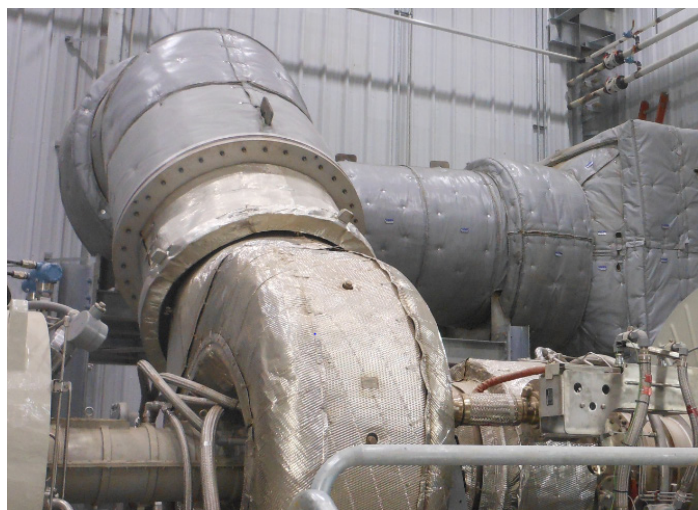
Gas Turbine Housing & Exhaust Ducting
