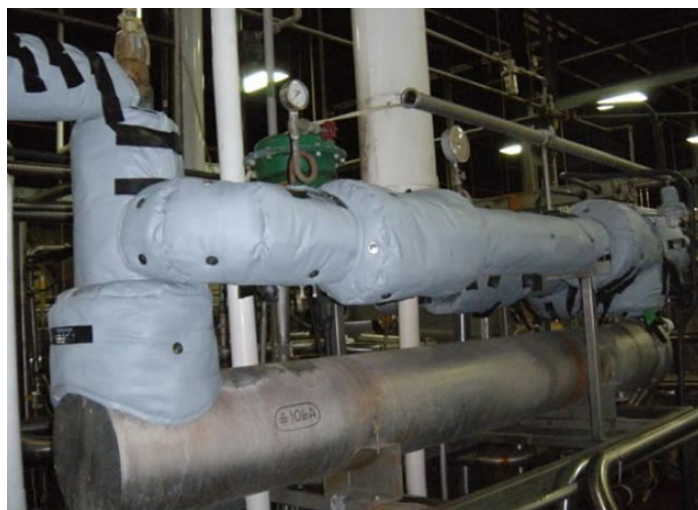
Steam Supply Control Valve Station Steam Pasteurizer
