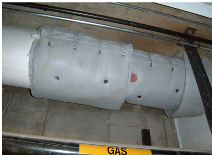
10” 300# Single Slip Expansion Joint Steam District Heating - Manhole
