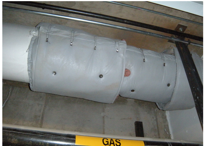
10” 300# Single Slip Expansion Joint Steam District Heating - Manhole
