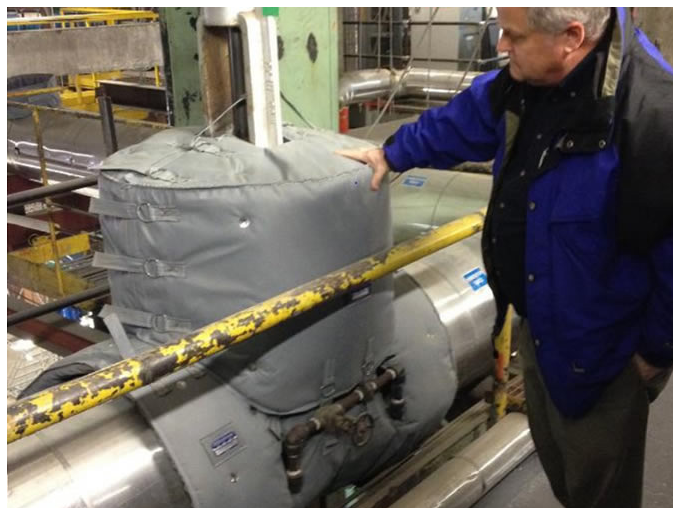
16” 300# Main Gate Valve - Steam Shut Off
