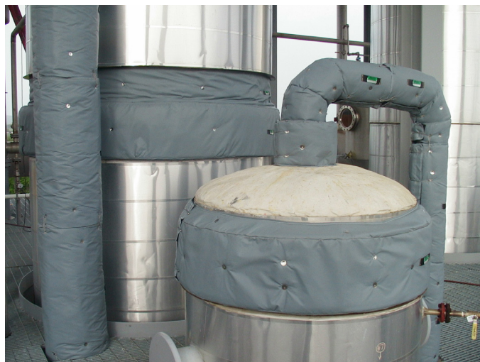
Process Distillery Vessels / Piping
