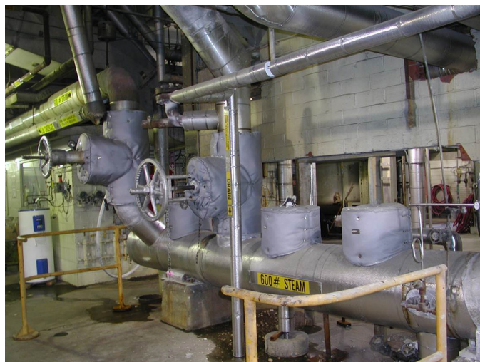
High Pressure Steam Header - Pulp & Paper Mill
