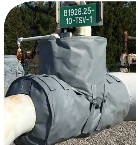
OIL PIPELINE - SHUT OFF VALVE
