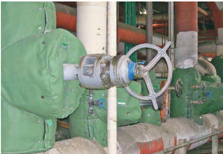
BOILER ROOM – MAIN HP STEAM HEADER GATE VALVES & VALVE BONNETS Design: LT450TT - 1.5" thickness Fastener: Stainless Steel Wiretwists and Velcro® Flaps
