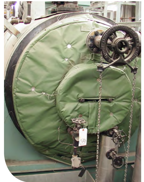
BOILER HEAD STEAM DRUM
