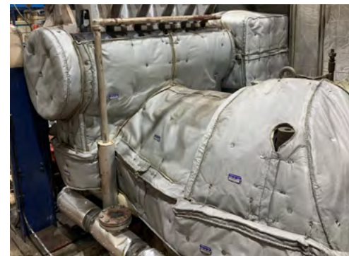
MULTISTAGE STEAM TURBINE Thermal Blanket Insulation Design: HT1100MSGM - 2" Thickness
