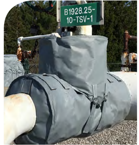
OIL PIPELINE - SHUT OFF VALVE
