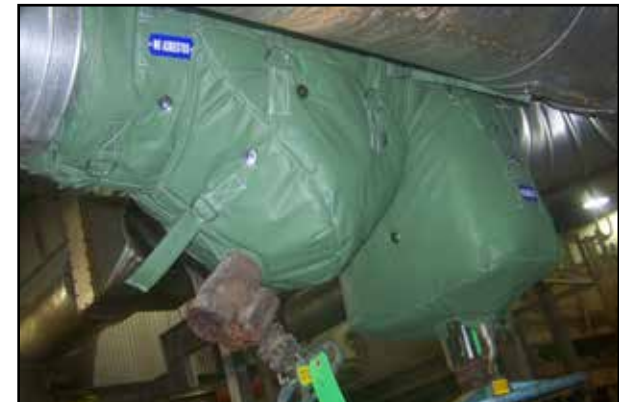
LT450TT HP STEAM GATE VALVE & STRAINER
