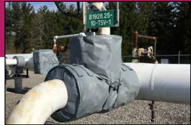
SSS-500-TAFT OIL PIPELINE - SHUT OFF VALVE
