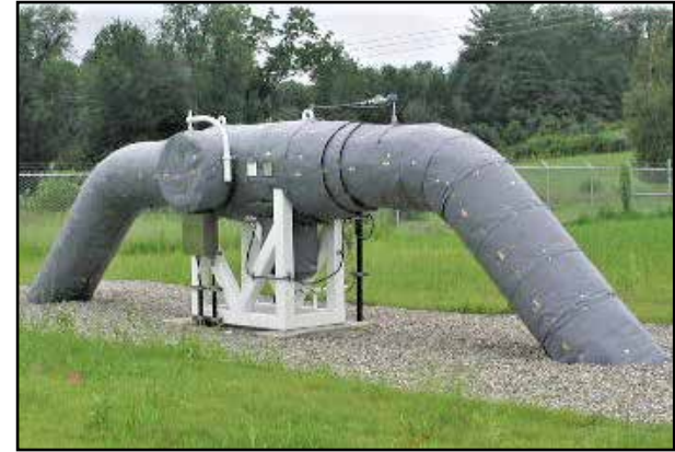
LT450-HES NATURAL GAS PIPELINE
